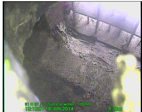
Photo: 140618_1010A-Survey.jpg 9.3m, Finish node type, manhole reference number: B1 ROAD GULLY
