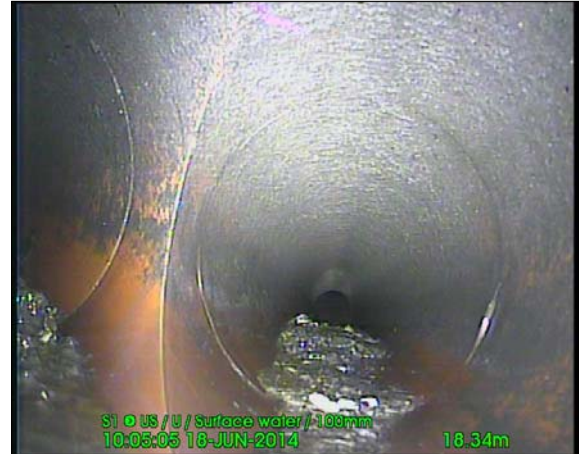
Photo: 140618_1005A-Survey.jpg 18.34m, Junction from 9 O'Clock diameter: 100 mm
