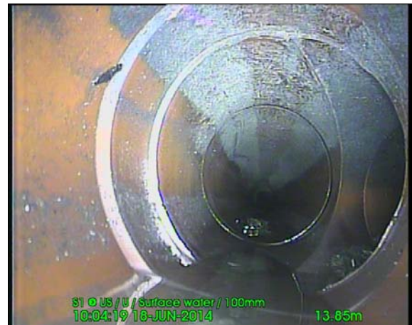
Photo: 140618_1004A-Survey.jpg 13.85m, Junction from 3 O'Clock diameter: 100 mm
