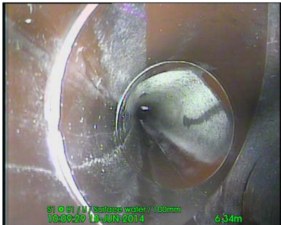
Photo: 140618_1009A-Survey.jpg 6.34m, Junction from 3 O'Clock diameter: 100 mm
