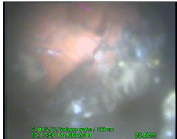
Photo: 140618_1017C-Survey.jpg 20.87m, Finish node type, manhole reference number US
