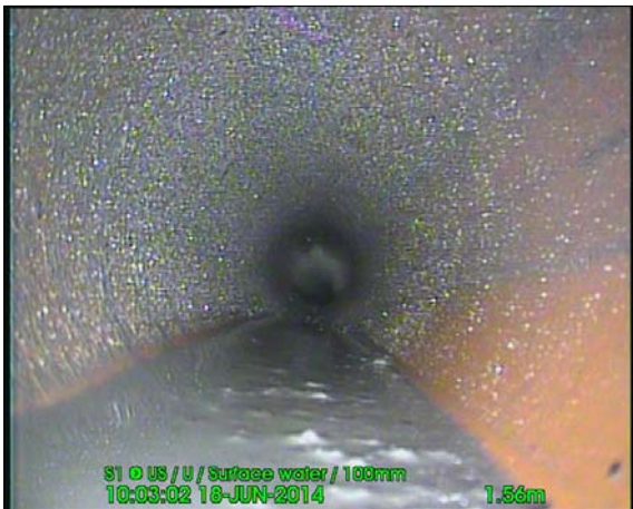
Photo: 140618_1003A-Survey.jpg 1.56m, Settled deposits, fine 15 % cross-sectional area loss S1 UNABLE TO JET SOAKAWAY FULL
