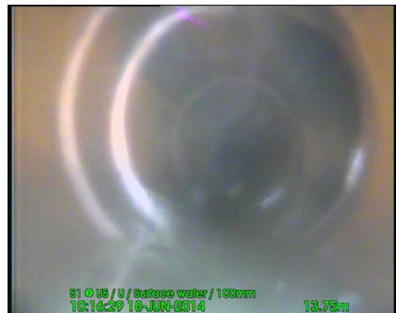
Photo: 140618_1016A-Survey.jpg 13.75m, Junction from 3 O'Clock diameter: 100 mm
